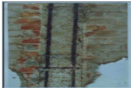
Spalled Concrete In Column
