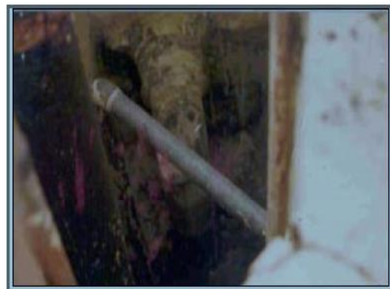
Isolated And Defective Drainage Line
