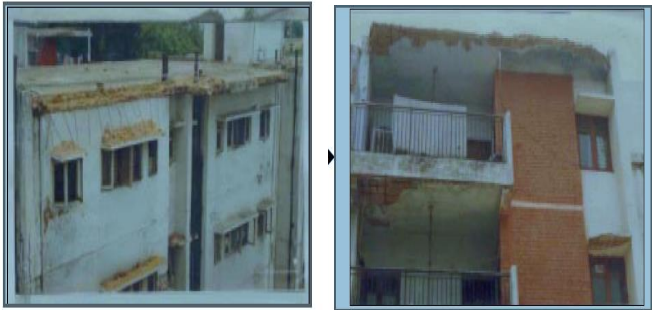
Detoriation & Damage of Building
