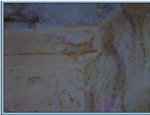
Damage Due To Leakage In The Building
