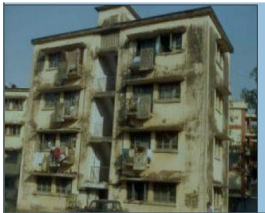
Deterioration Of Building Due To Ageing
