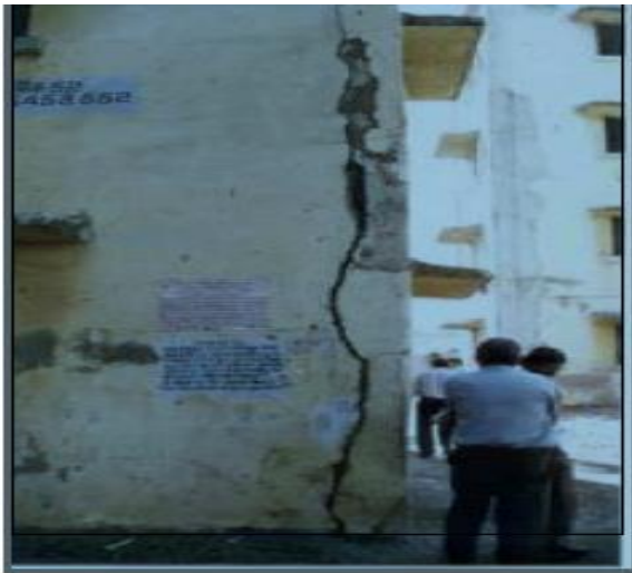
Cracks in Column
