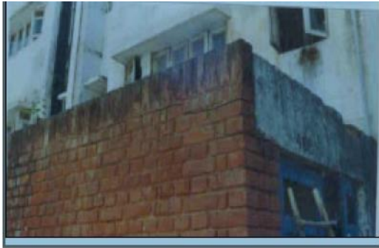
Cracks In Masonry
