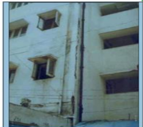
Cracking Of Column At Plinth Level
