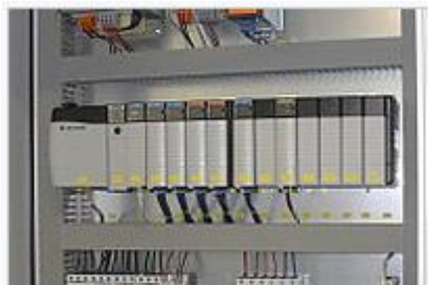
Fig No 3 Allen-Bradley PLC installed in a control panel
