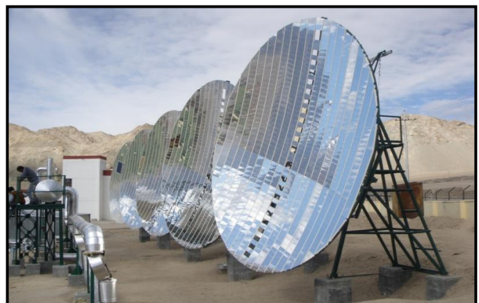
Fig-5: Actual photograph of solar field for an auto ancillary company in north India.
