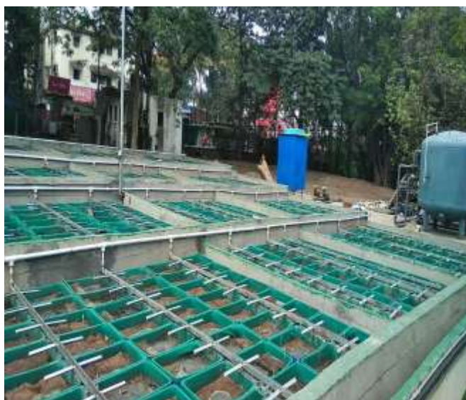
Fig -1: Showing actual Tiger biofilter plant at Sahakarnagar
