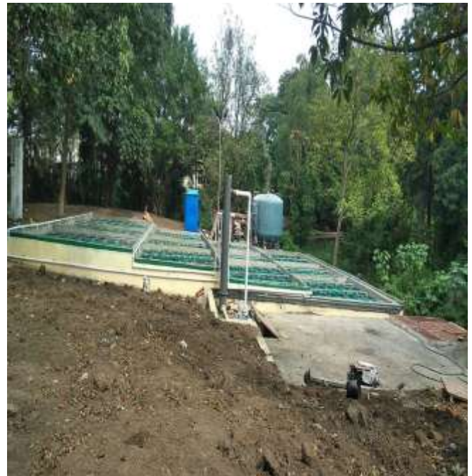
Fig -2: Showing actual Tiger biofilter plant at Sahakarnagar
