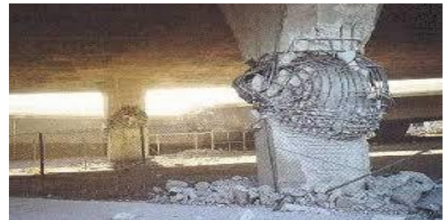
Figure 3.1 Failure of RC column
