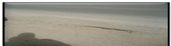
Figure (2): Lane Shoulder Drop Failure in Study Area
