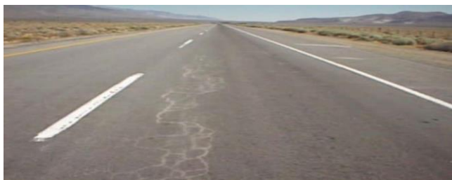
Figure (3): Alligator Cracking Failure in the Study Area
