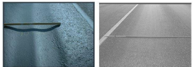
Figure (1): Rutting Failure in Study Area
