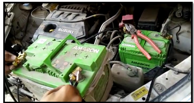
Fig -3: Lead Acid Battery
