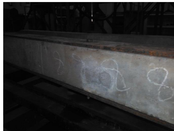
Fig 3: Retrofitted with one plates top and one plate base of the beam
