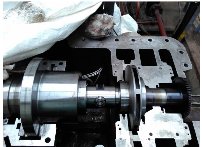
Fig -1: Turbine front end journal bearing
