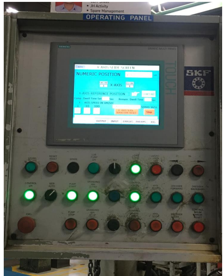
Figure -3: Siemens Multi Touch Panel
