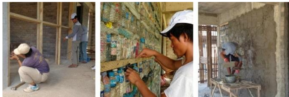
Fig.2: Vertical Bottle Wall Construction- Wall Frame, Wire Mesh filled with Bottles and Final Plastering Process
