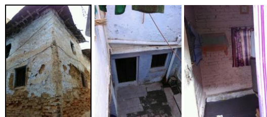
Figure 4: Housing Conditions of weavers
