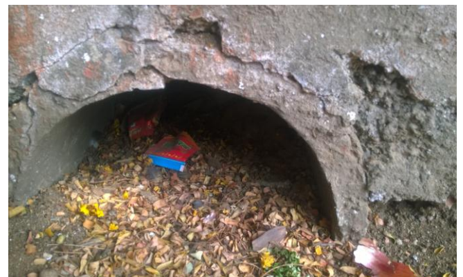
Fig -4: Sedimentation in storm sewer
