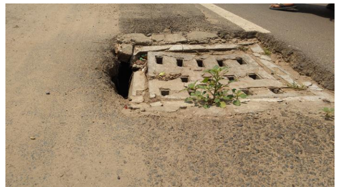
Fig -3: Condition of Manhole
