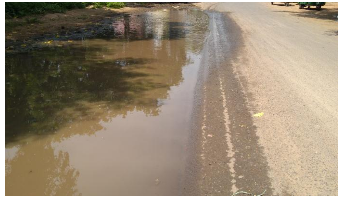
Fig -2: Stormwater Problem
