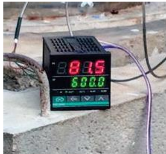
Fig-3: PID Temperature Controller
