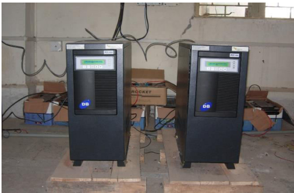
Figure 4 Power Control Units setup for Solar & Wind
