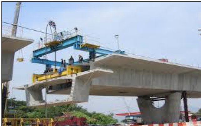
Fig -2: Cantilever construction of pre-stressed concrete box-girder bridge decks with pre-fabricated segments (Source: Design guide-Pre-stressed concrete cantilever bridges)
