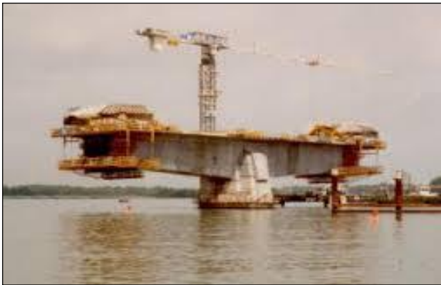
Fig -1: Cantilever construction of pre-stressed concrete box-girder bridge decks with cast-in-situ segments (Source: Design guide-Pre-stressed concrete cantilever bridges)
