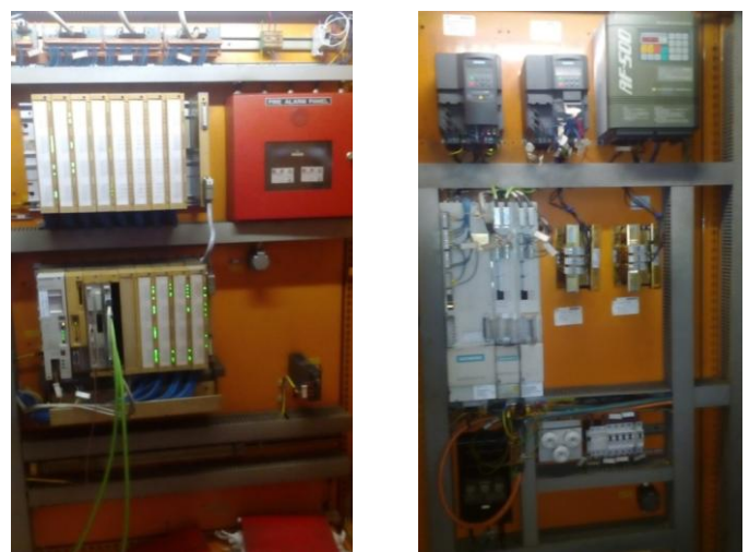
Fig-3: Electrical Control panel of Top Surface Grinding Machine
