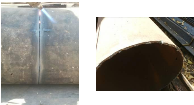
Figure D- Side and front view of MS pipe during and after cutting
