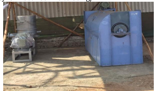
Fig-3: Shredding Machine in RESIL, Jejuri
