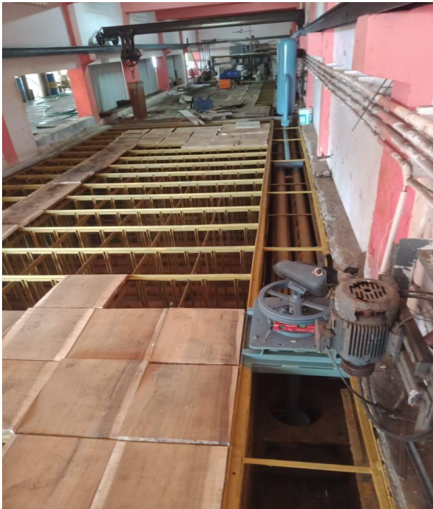
Fig-2: A typical ice plant chilling tank.
