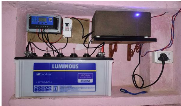
Fig -11: Complete Residential Installation Battery, Charge Controller, Inverter Unit and AC Output
