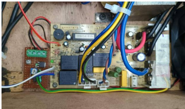
Fig -1: Modified UPS Control Board (100754-01G) with Custom Add-on PCB
