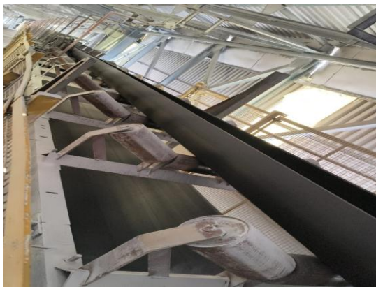
Figure 3: Central long-run view showing the distributed nature of conveyor rotating elements
