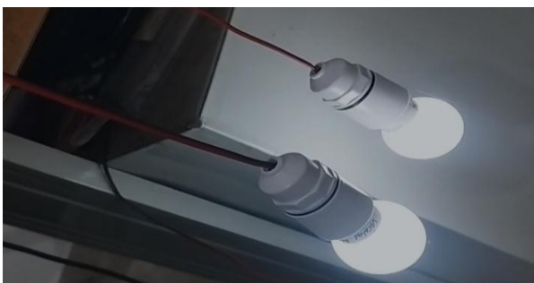
Fig 4. Lights are switched ON based on detection results
