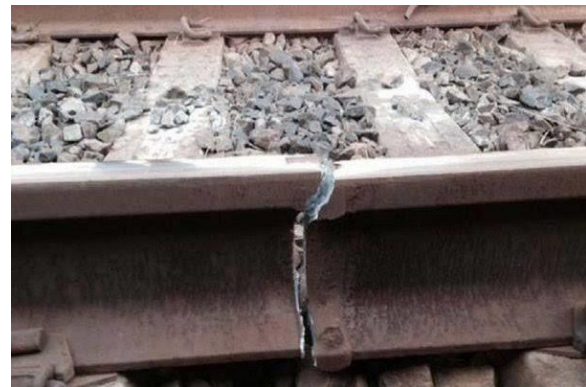
Fig -1: Crack in Railway Track
