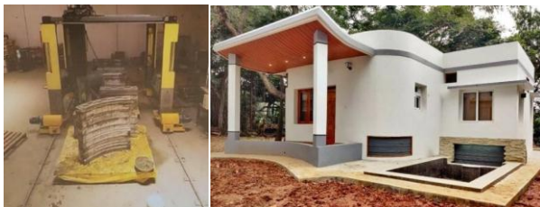
Fig -5: India's first Industrial size 3d Concrete printer at IIT Madras by TVASTA & India's first 3D Printed house at IIT Madras (3DParts printed by Offsite printer, transported and assembled at site.)
