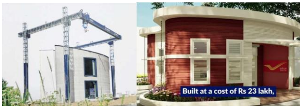
Fig -4: COBOD gantry type printer (BOD 2) & India's first 3D printed post office building at Bangalore made with COBOD printer, constructed by L & T. 1000sqft in 45 days, Crew of only 5 peoples. Cost 23 lakhs. Life span 50 to 100 years
