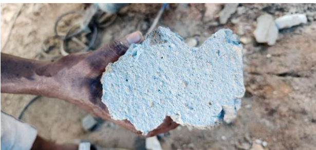
Fig -42: Cross section examination. No serious cold joints, shrinkage cracks or voids found, chance of porosity
