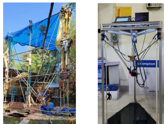
Fig -8: Delta 3D printer at CUSAT, Kochi & Delta 3D concrete printer at Minvayu, Auroville
