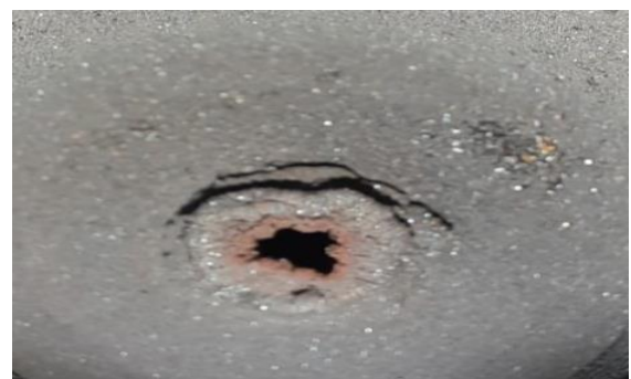
Fig1. Orifice Choking due to Crud accumulation
