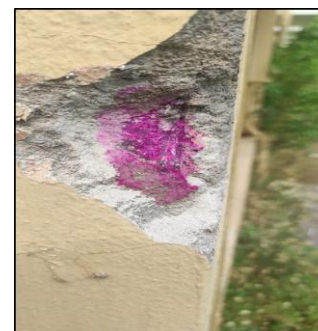
Fig.4 Carbonation test on RC beam
